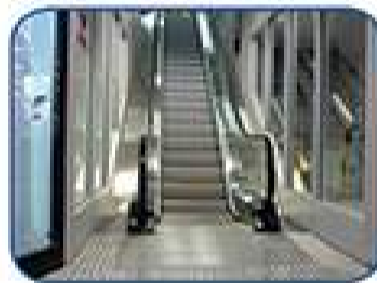
Bạc thang cuốn Handrail escalator
